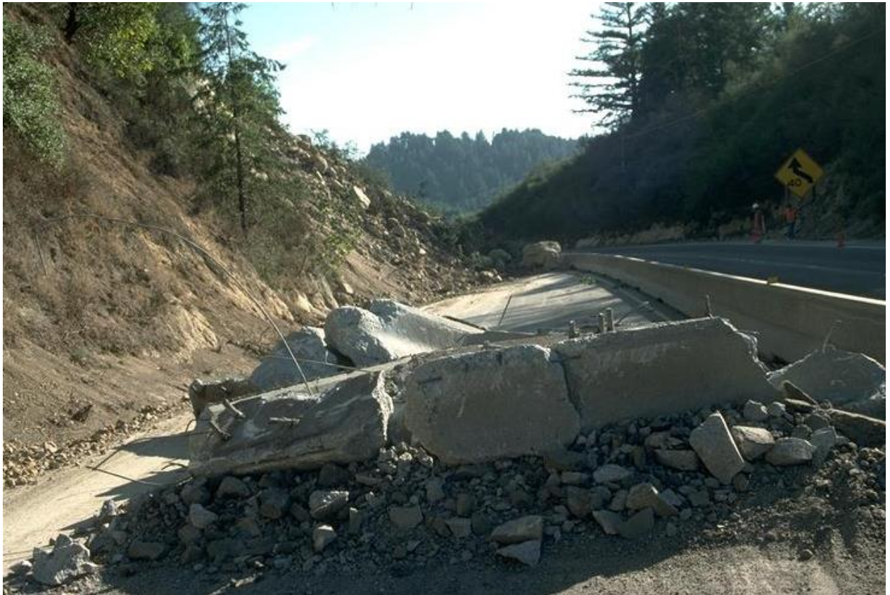
Figure 2.2: Broken chunks of concrete blocks on a Highway Anderson 1997.
