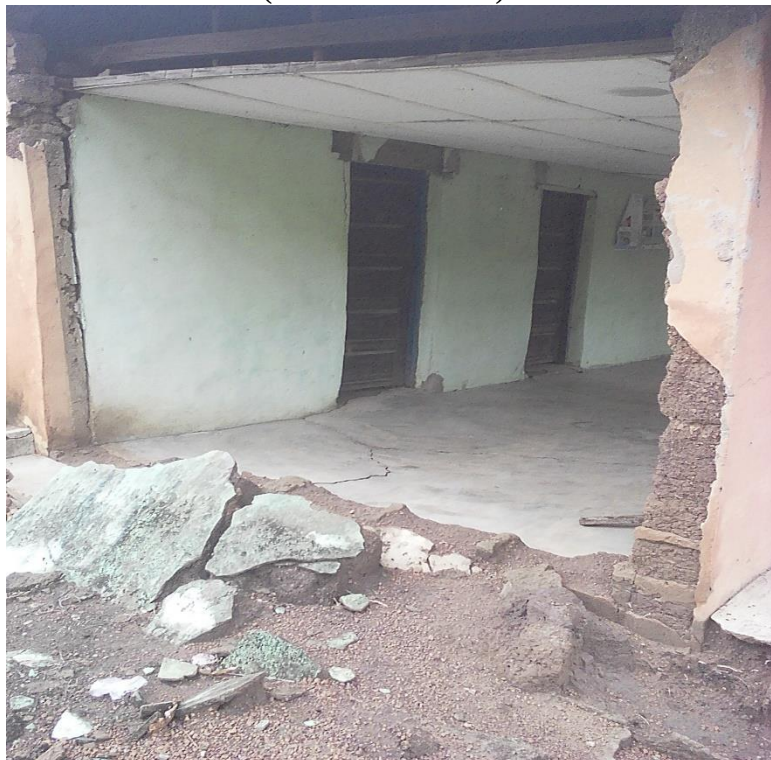
Figure 18: Dilapidated side of the building of Adankari Health Clinic – a relic of the outcome of the 1989 NPTA workshop. (Researcher: 2017)
