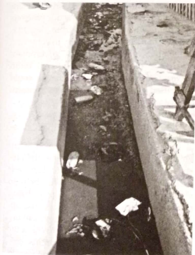
Plate 6: Blocked and foul-smelling drainage, Adangba. Source: Field Survey, 2017.
