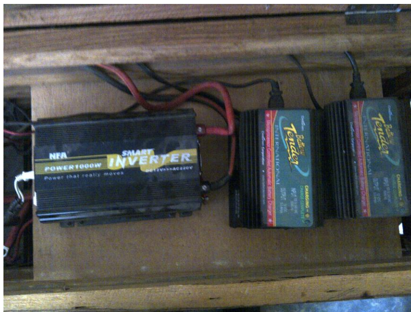
FIGURE 3(b): INVERTER AND BATTERY CHARGERS USED IN THE SYSTEM
